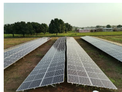
Mali: Rural Electrification
